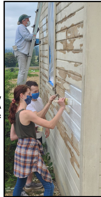
Treasurer Connie Zimmerman, intern Taylor Hill and friend Hendy Conlan scrape to the original cedar siding
